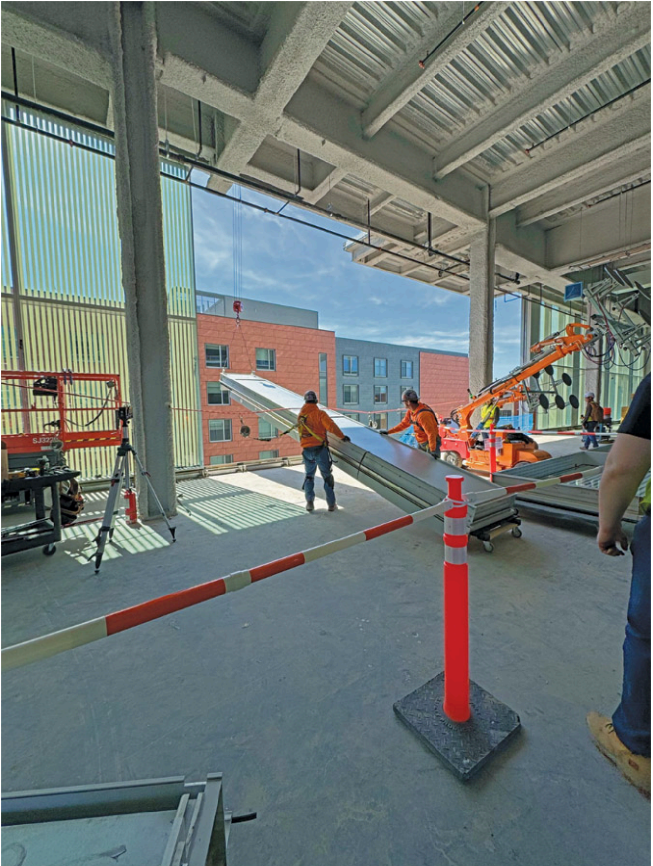
Reflection Window + Wall installs its RWW 8000 System at Hyde Park Labs at Harper Court in Chicago. Photo courtesy of Reflection Window + Wall
