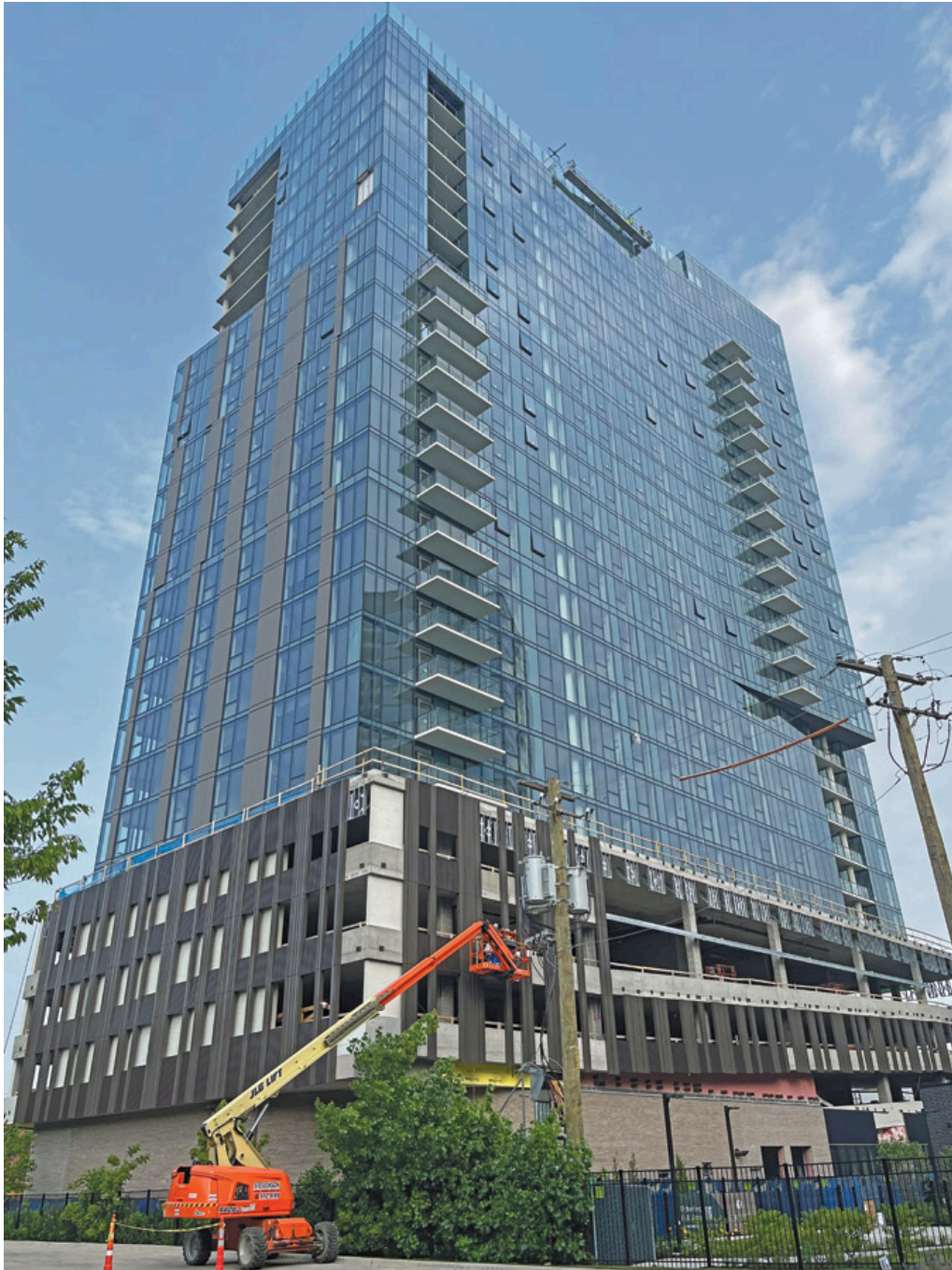
The company worked on a 27-story residential tower in Chicago's Lincoln Park neighborhood. Photo courtesy of Reflection Window + Wall
